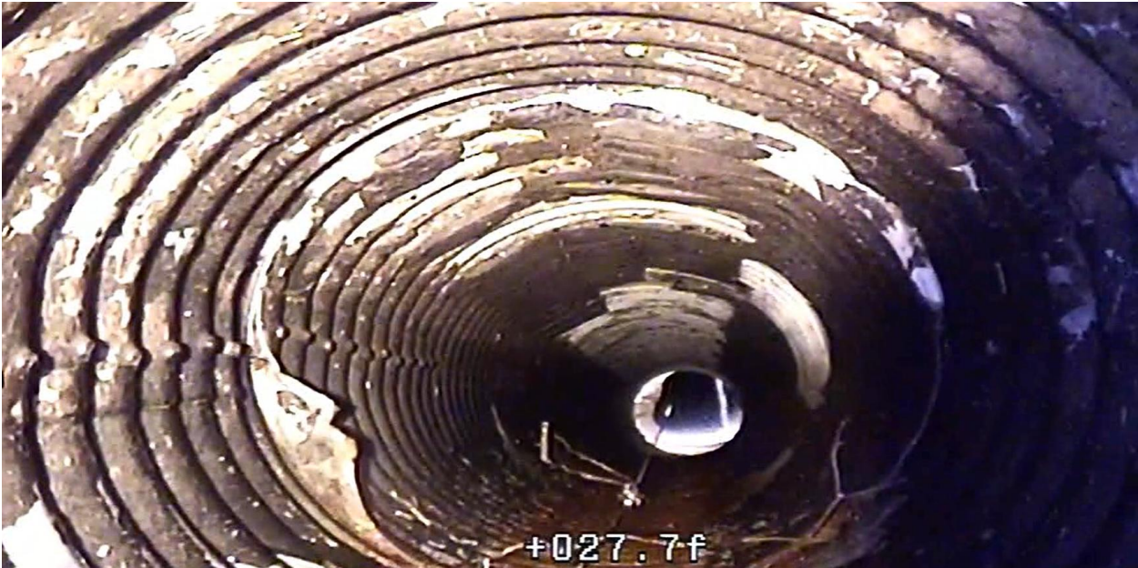
Holes in pipe and bent metal.
