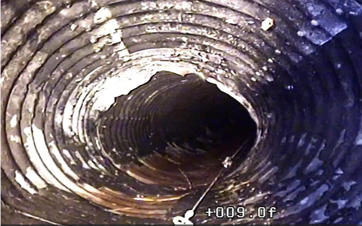
Pipe is compressed to an oval. Bent metal at pipe joint won't allow CIPP or Sliplining.
