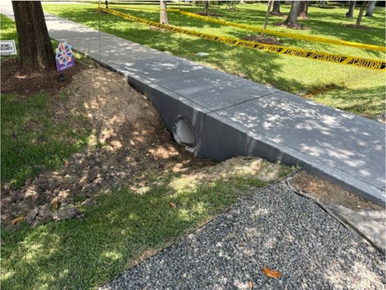
Figure 1 New Walkway and Pipe (Needs Restoration)
