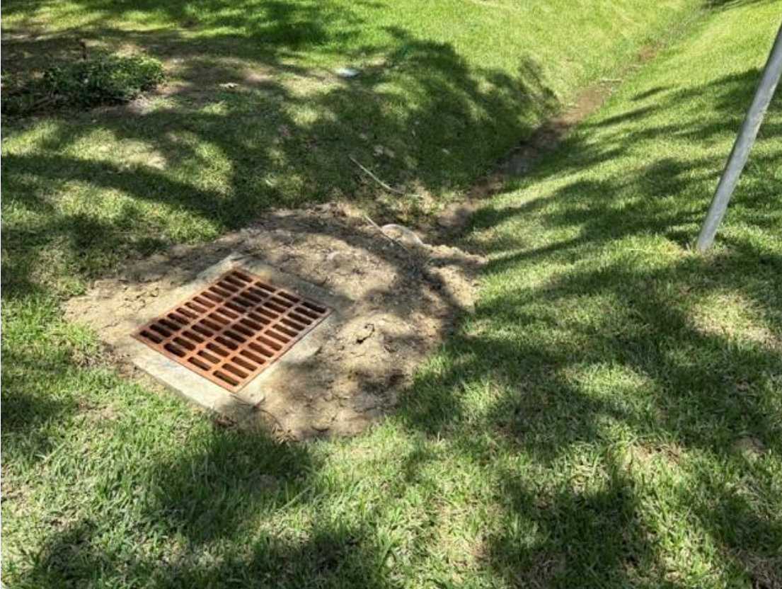
Figure 2 New Inlet at 609 Lindenwood (Restoration Needed)
