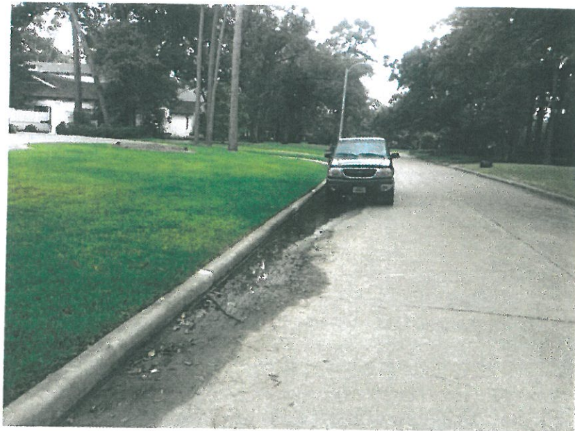
Location No. 20 – 19 & 23 Willowron Drive (2 of 2)
